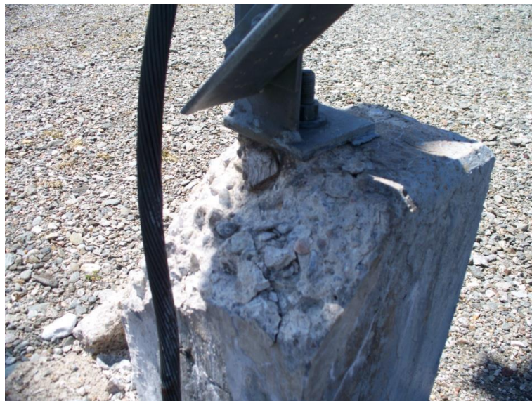
Figure 15: Structure B1T1 Bottom Brook Terminal Station
