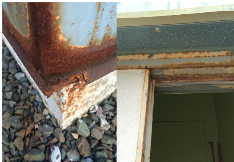
Figure 18: Building Exterior Cladding and Exterior Doorways Displaying Severe Rusting and Deterioration
