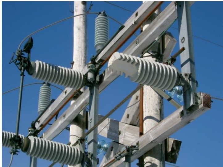
Figure 4: Broken Insulator on 69 kV Disconnect Switch
