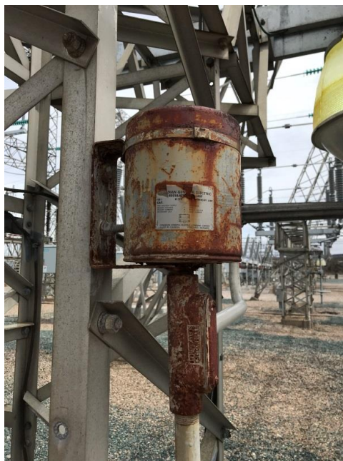
Figure 13: Corroded Ballast Requiring Replacement
