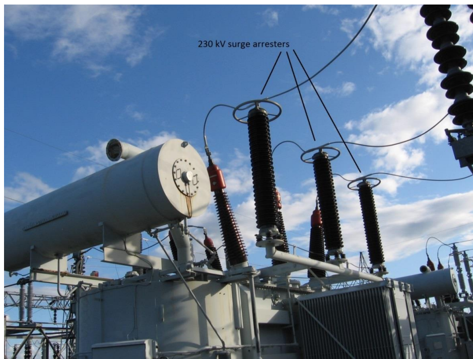
Figure 5: Western Avalon Terminal Station Transformer T3 230 kV Surge Arresters
