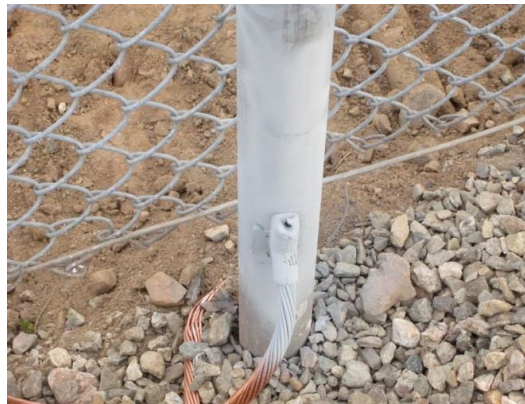
Figure 7: Typical Grounding Connection on Terminal Station Fence
