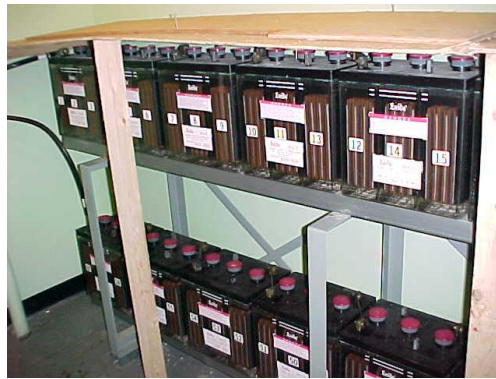
Figure 11: 125 Vdc Terminal Station Battery Bank
