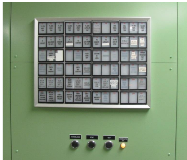
Figure 20: Annunciator Commonly Found in Hydro Terminal Stations
