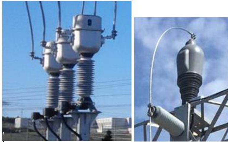
Figure 1: 69 kV CT (Left) and PT (Right)
