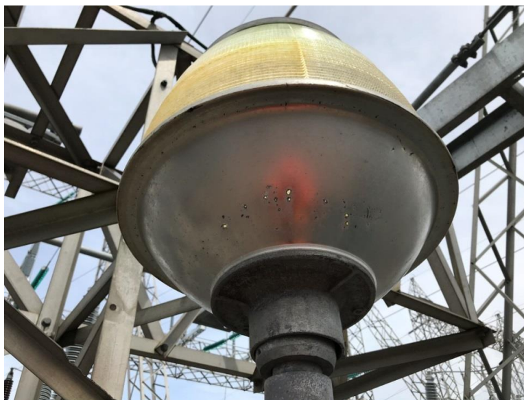
Figure 14: Light Fixture Showing Perforations due to Corrosion, Enabling Moisture Ingress
